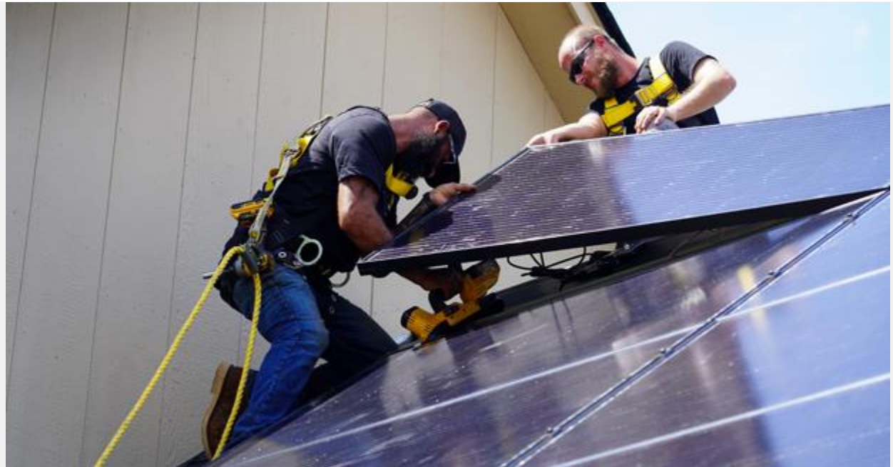
Workers for EightTwenty install solar panels on the new farmers market operated by Restore OKC in Oklahoma City. (Courtesy photo)
